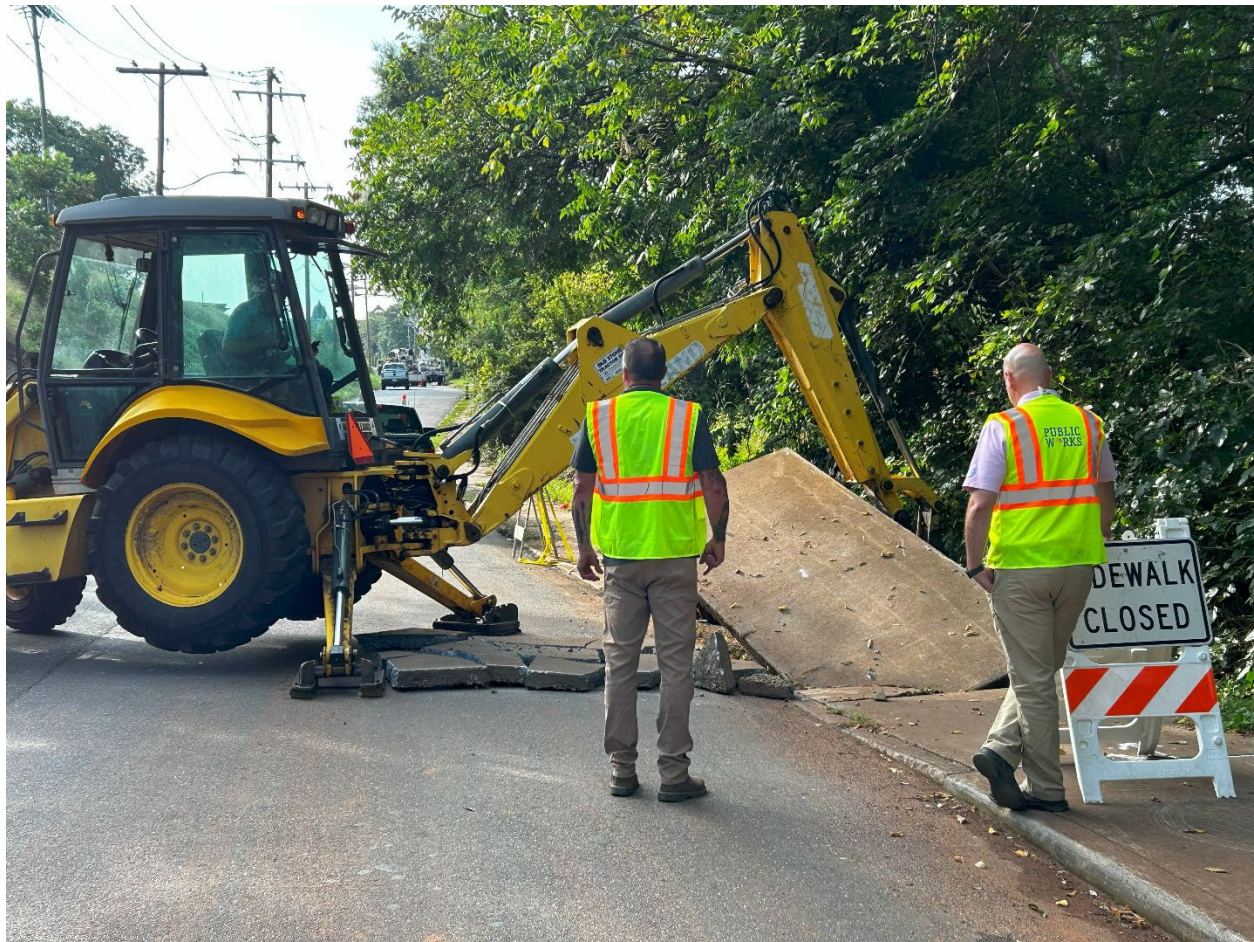
Stormwater crew accessing partial road washout.
