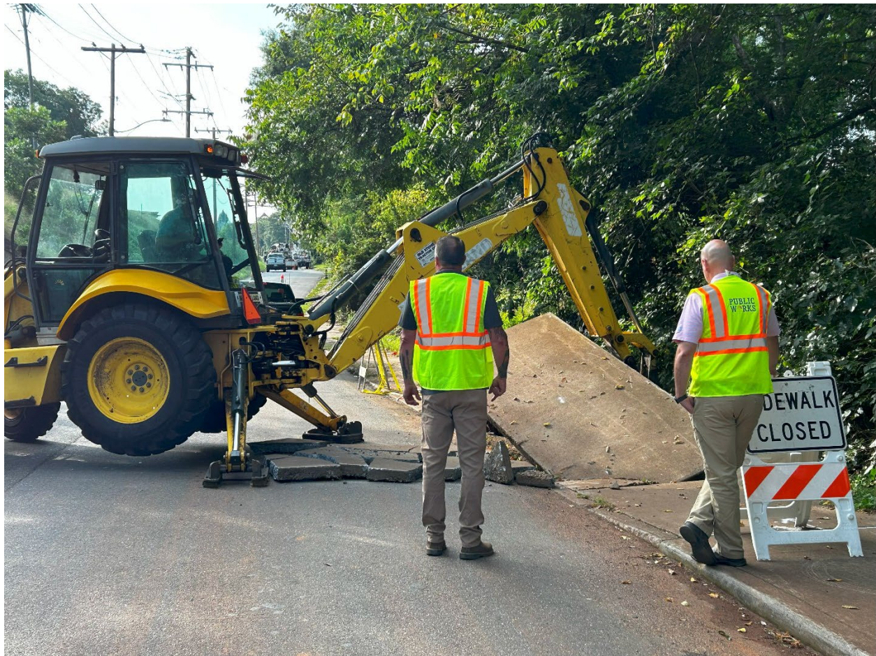
Stormwater crew accessing partial road washout.
