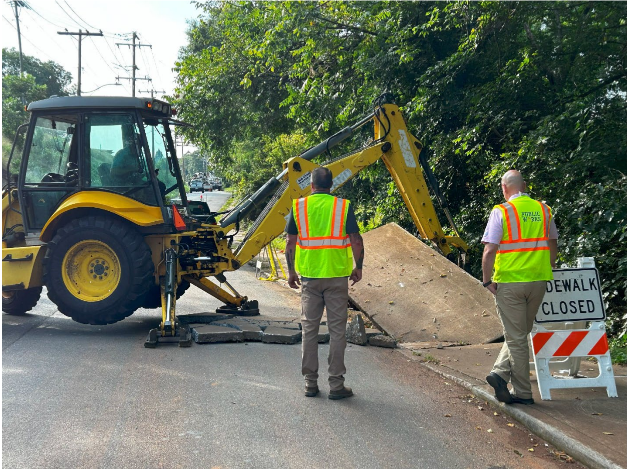
Stormwater crew accessing partial road washout.
